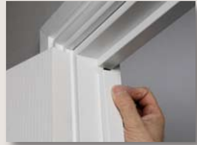
STEP 9: Fix the vertical door stops in position, using an appropriate glue if required, checking that the fitting is consistent on all edges.
