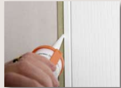
STEP 12: Apply an appropriate adhesive to the groove in the lining that the architrave will be positioned in.
